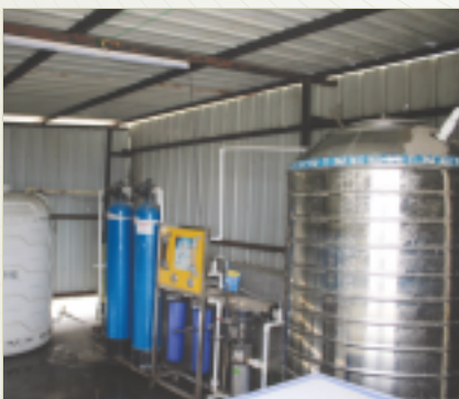
RO Water Plant
